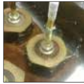
Leaking valve during cold temperature testing
